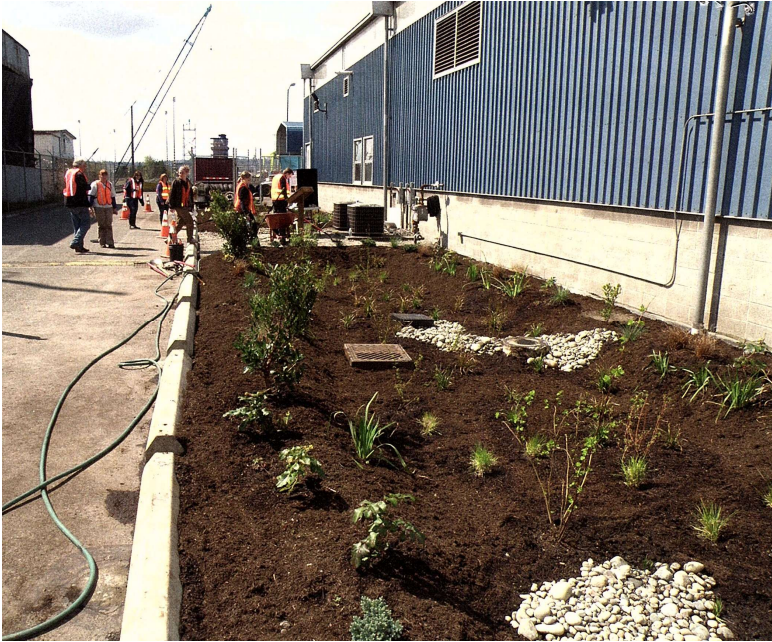
Photo 103: Rain gardens can be expanded for industrial and commercial areas. They can be constructed within and adjacent to impervious surfaces such as parking lots. In some cases, rain gardens can store and treat up to 10% of the parking lot runoff.
